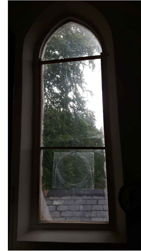
Detail of "temporary" window to be replaced with a new diamond zinc framed window glazed with original glass which has been kept in storage.
